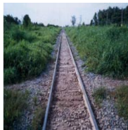
Figure 9 Mud pumping appeared along Baeng Pra - Pitsanuloke
