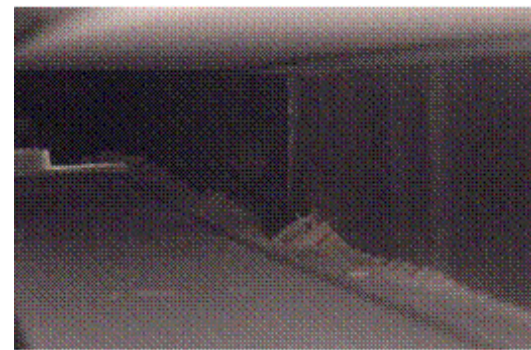
Figure 9. Failure Mode for Crowned Deck under Fatigue Loading
