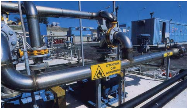
Fig. 5. Photo of the technological Area.
