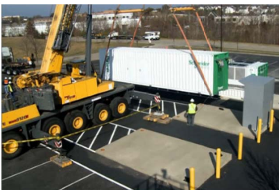
Figure 8 Mobile data center
