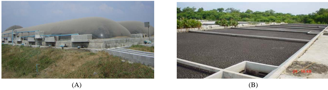
Figure 4. (A) CMU-UF digesters from actual location, (B) Sand-bed solar-heated sludge drying units (courtesy of ERDI-Nakornping, CMU).
