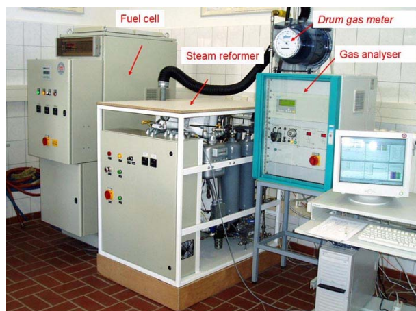
Figure 1. PEM fuel cell test stand for biogas at ATB (1 kW_{el} )
