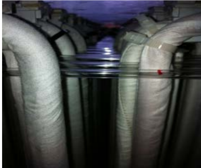
Fig. 5. Perforated desiccant pipes penetrating the tube-bundle.
