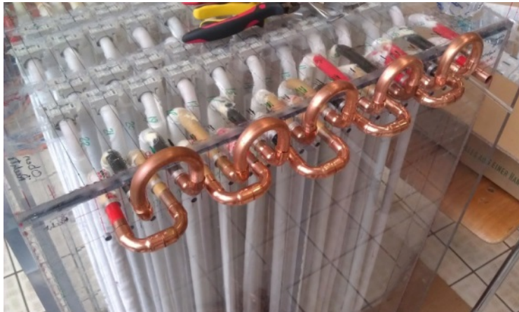
Fig. 7. Solder joints and the pipe connectors.
