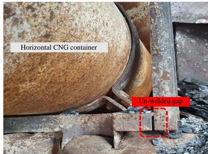
Figure 13 Poor mounting structure of CNG container near dispensing unit.
